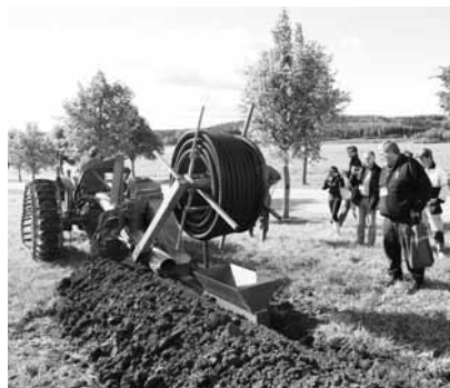
Demonstration of drainpipe installation equipment at Kalnes Agricultural College (Photos by Toomas Tamm).
